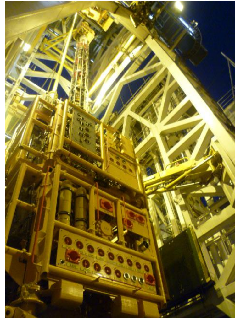
7 3/8" SIL assembly (comprising Stuffing Box/OWL; Riser (lubricator) EDP, LRP & spool connector > client TRT) positioned in the MPT prior to deployment
